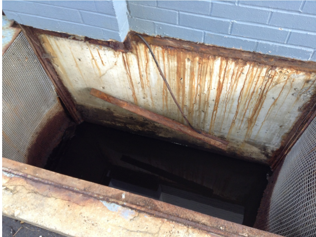
Car wash sump covers are submerged in approx. 1.2m liquid. Metal bracket fixed to car wash wall severely corroded and piece is hanging suspended at side of pit
